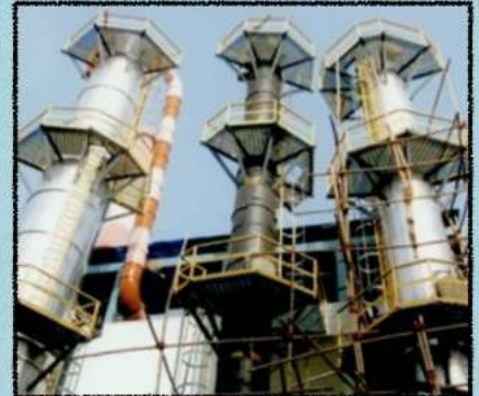
ERCON FRP Cage Ladders, Platforms complete with base structure, gratings & hand rails on chimneys of an industry.
