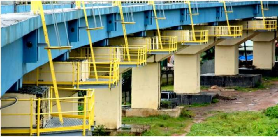
Vaillarpadam Railway Bridge, Kerala, India, Ercon GRP Platforms with Cage GRP Ladders, Handrails, Structure & Gratings
