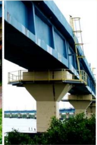
GRP - Bearing Inspection Platforms
